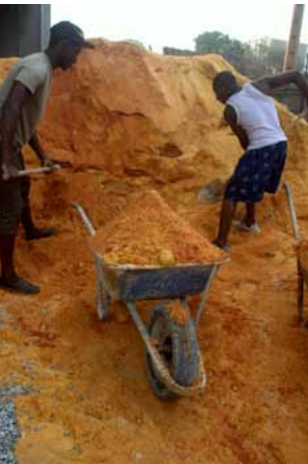
Construction work in Conakry, Guinea, supports early economic recovery. (Photo: UNDP Anne Kennedy)
